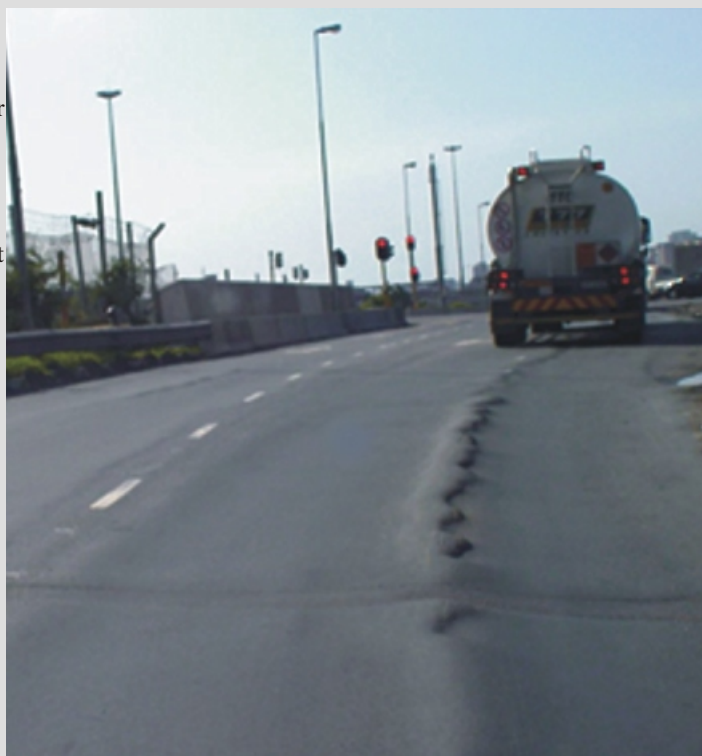
Figure 3. Current condition of a road surfacing outside Durban harbour, where HiMA will be put to the test
