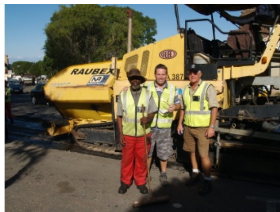
National Asphalt's Mike Walsh and SSI's Peter Jerome discuss paving of WMA base in Malvern with a paving crew member
