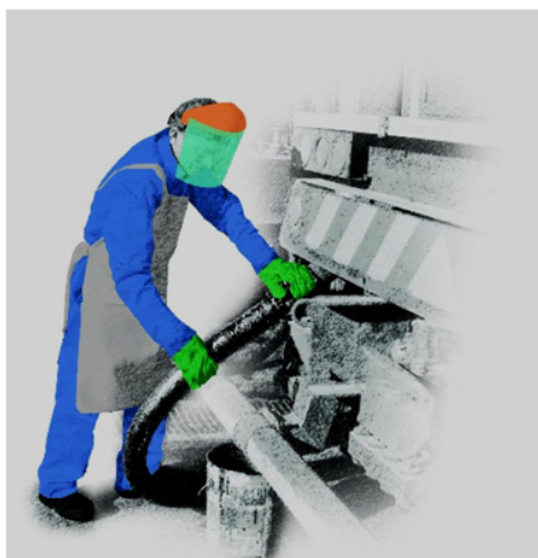
Figure 5: Safe handling of bitumen on site with the proper personal protection equipment
