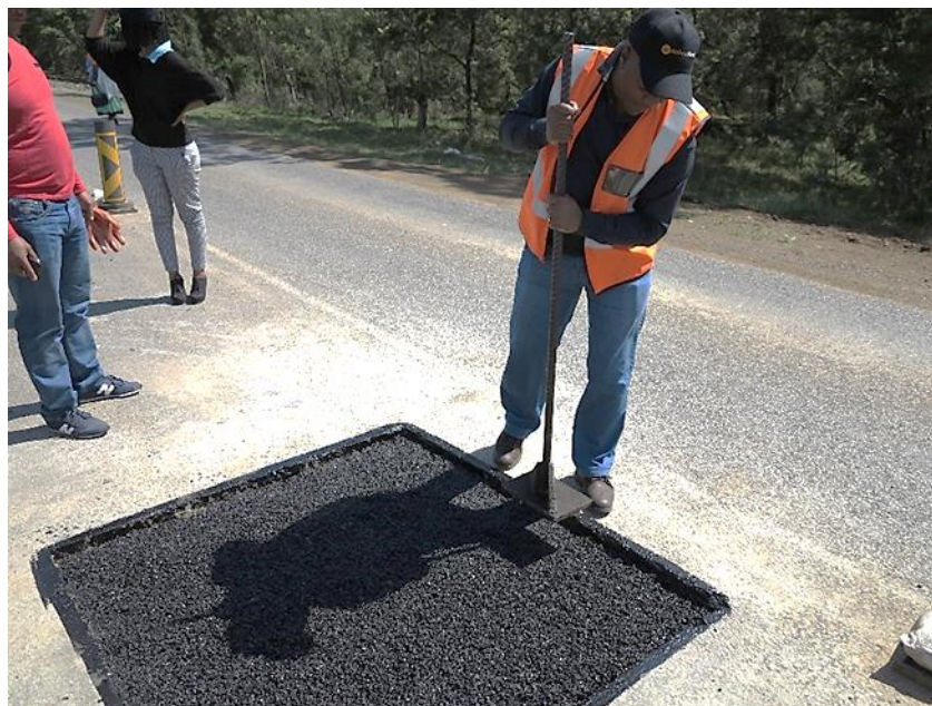
Photo 8: Large pothole prepared for repair
