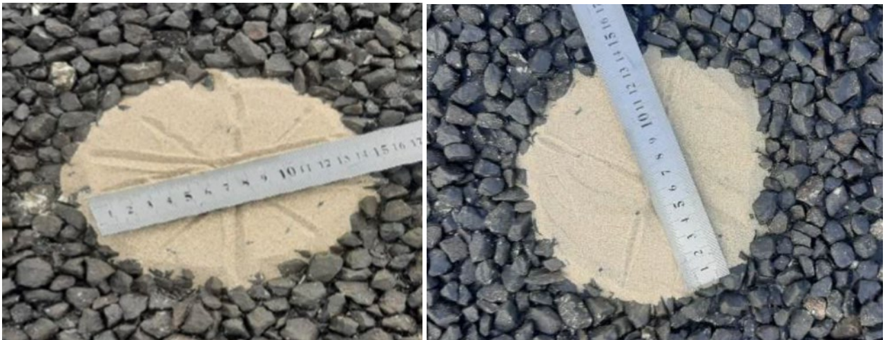
Figure 6 Sand not spread sufficiently
