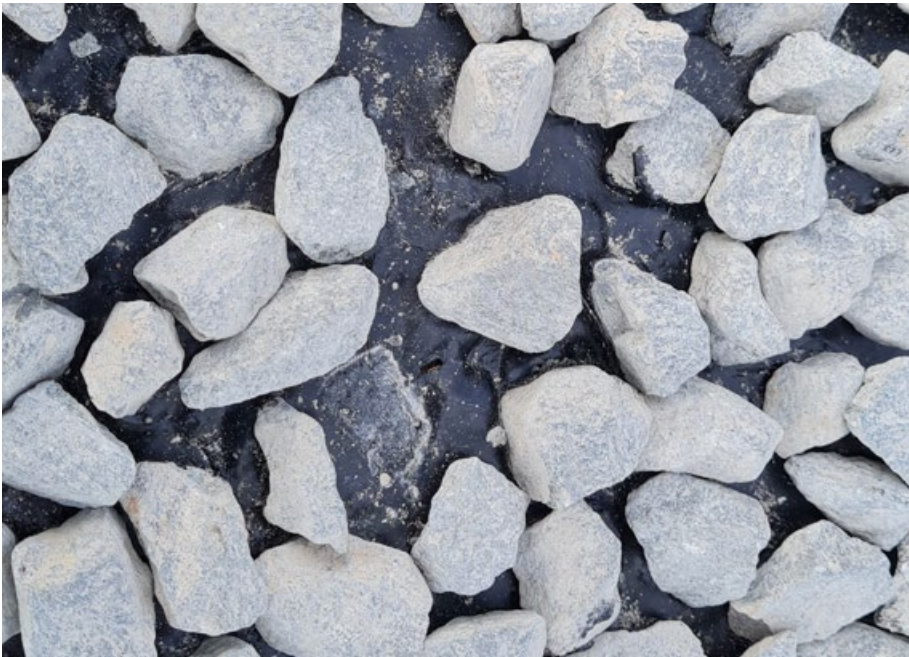
Figure 37 Poor adhesion of quartzitic stone to polymer modified emulsion
