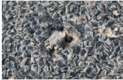
Figure C 8 Base Aggregate Visible in Seal Structure
