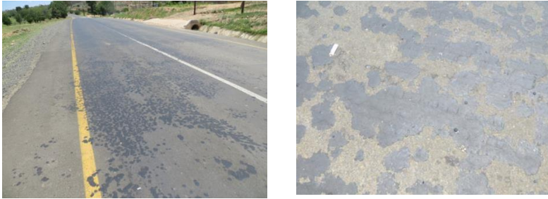
Figure H 29 Bitumen from Bleeding Cape Seal Migrating through 30mm Asphalt
