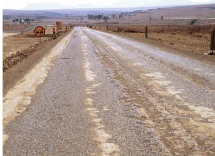
Figure D 10 Poor Performing Single Seal
