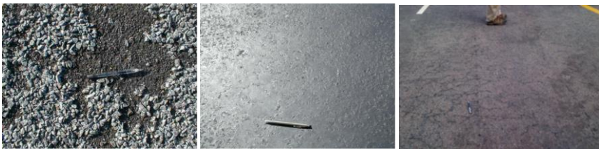
Figure C 1 Distress Defining "End-of-Life"
