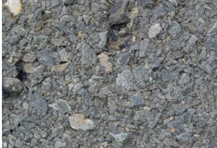
Figure D 8 Dry Porous Surfacing Requiring Rejuvenation
