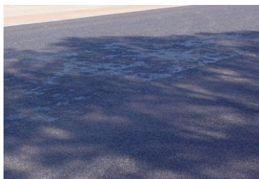
Figure E 22 Aggregate Loss due to Cold Shady Area
