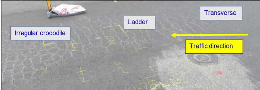
Figure C 27 Crack Development and Progression in Stiff Cape Seal with Modified Binders
