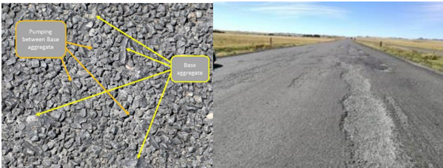
Figure C 10 Base Aggregate in Contact with Tyres and Subsequent Failures
