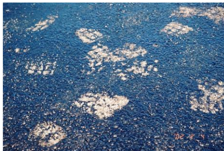
Figure F 40 Diluted Cationic Spray Grade Emulsion Not Penetrating
