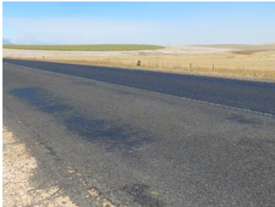
Figure H 19 Stripping and Fattiness on a Newly Constructed 14 mm Seal
