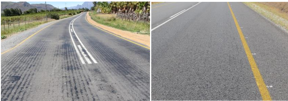
Figure F 13 Effects of Poor Transverse Distribution
