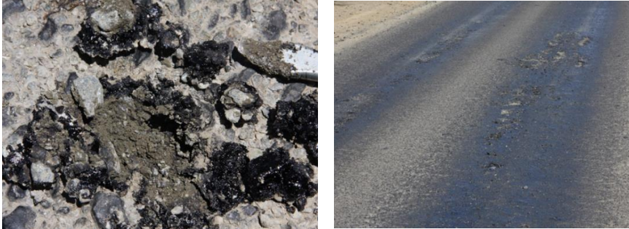
Figure H 3 Bleeding as a Result of High Base Moisture
