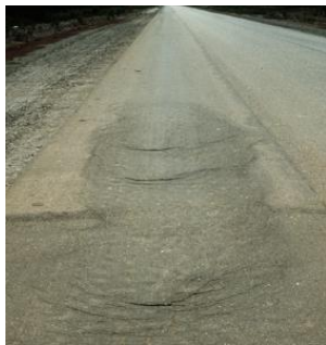
Figure C 16 Shear and Slippage of a Microsurfacing on a Smooth Base
