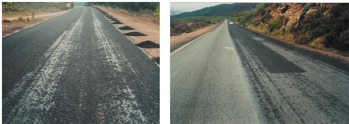
Figure H 23 Severe and Complete Loss of Aggregate
