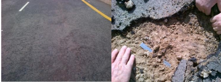
Figure C 6 Cracking of a Cape Seal on a Thin Soft Layer
