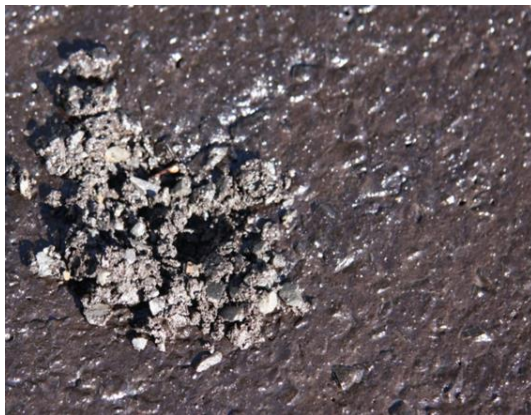
Figure F 38 Emulsion Segregated from Slurry Mix due to Too Early Rolling
