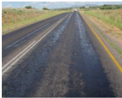
Figure H 4 Bleeding as a Result of Volatile Evaporation from Rejuvenation Treatment
