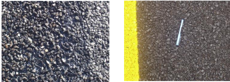
Figure H 25 After Application of Coarse Aggregate and the Final Repaired Surface
