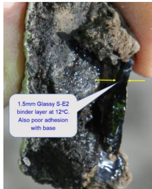
Figure C 28 S-E2 Binder Layer with Poor Adhesion to Base and Seal Aggregate
