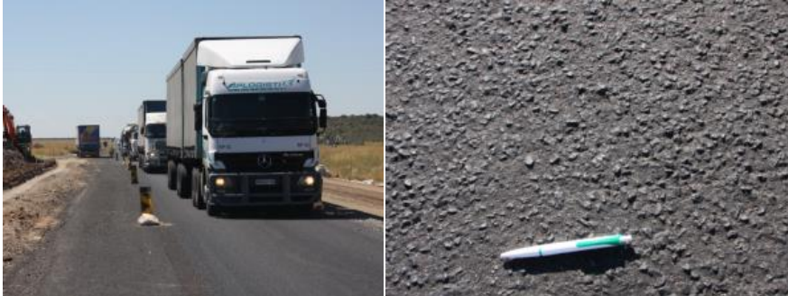
Figure D 13 Temporary 10 mm Cape Seal after 1 year
