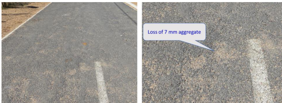
Figure C 13 Loss of 7 mm Aggregate on a S2(14/7) Double Seal due to Poor Compaction
