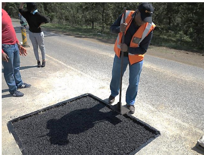
Photo 8: Large pothole prepared for repair
