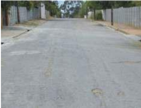
Photograph 18: Impact of poor transverse distribution
