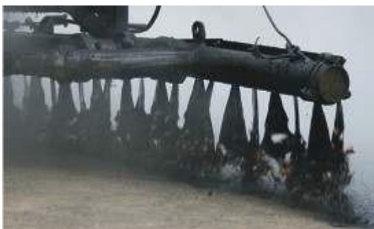
Photograph 17: Poor spray-bar distribution
