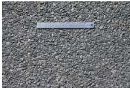
No defects apart from dry and brittle
