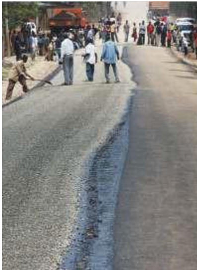
Photograph 14: Damage by chip spreader
