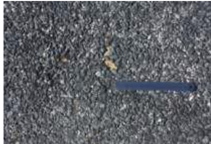
Small surfacing failures occur
