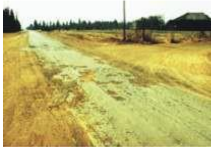
Disintegration of surfacing at intersection within 6 months
