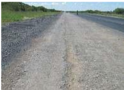
Base damage due to trafficking
