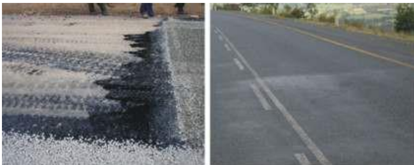
Photograph 15: Transverse joint problems
