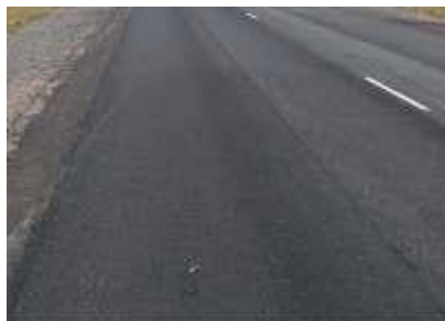
Microsurfacing applied (minimum 8 mm) allowed quick opening to traffic and can serve as initial seal for several years
