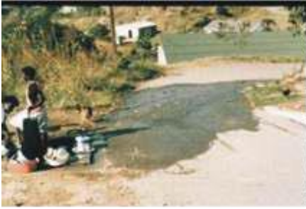
30 mm asphalt on steep grades. Water and chemical erosion measured at 5 mm/annum
