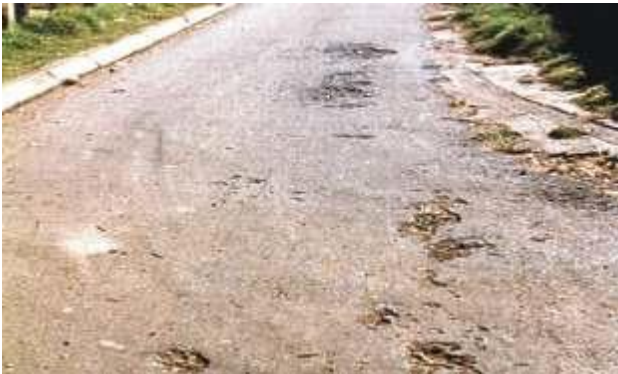
13,2 mm plus 6,7 mm double seal after 3 years on steep grade in urban developing area. Soil wash and high binder 10 years
