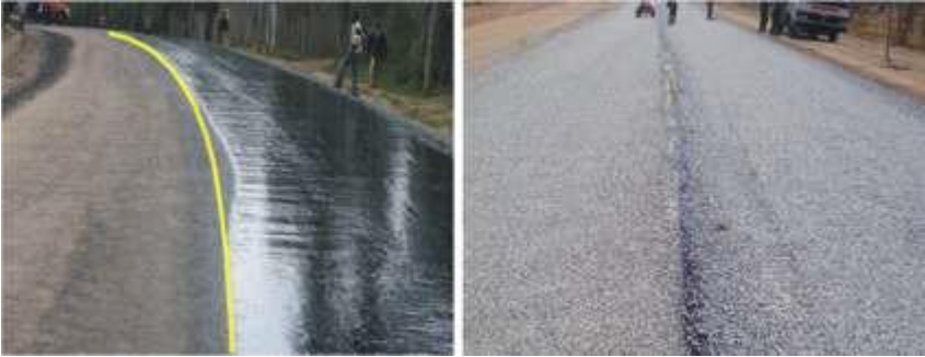
Photograph 13: Poor longitudinal joint construction
