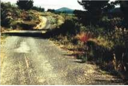
13,2 mm single seal after 3 years. Binder content too low and construction defects evident
