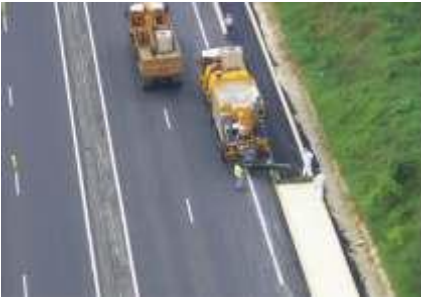
Photograph 11: Coloured slurry on cycle lane
