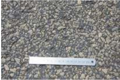
Aggregate loss and small surfacing failures identify the need for resurfacing
