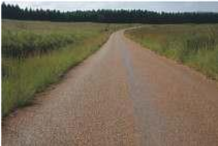
13,2 mm single seal after 25 years on properly constructed base and with high application rate
