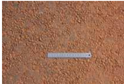
No defects apart from dry and brittle binder irregularities in base
