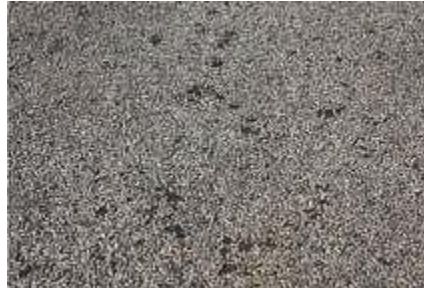
Aggregate loss evident
