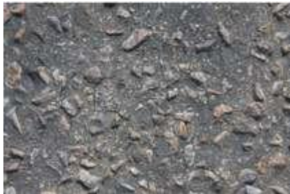
Oxidation/hardening of the binder and fine cracking identify the need for resurfacing
