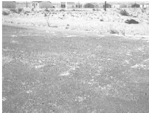
Ravelling of sand asphalt
