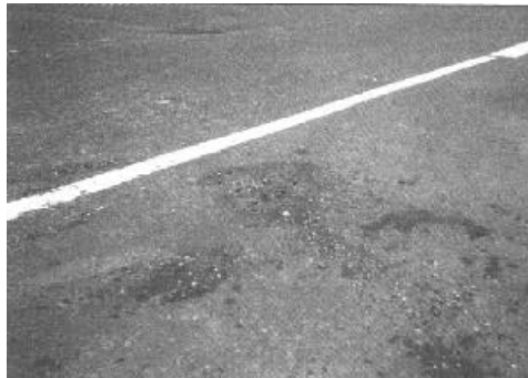
Disintegration of sand asphalt
