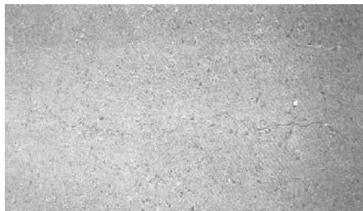
Longitudinal cracking in sand asphalt
