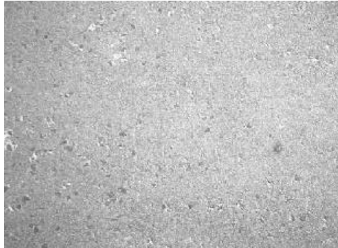
Compaction cracking in sand asphalt
