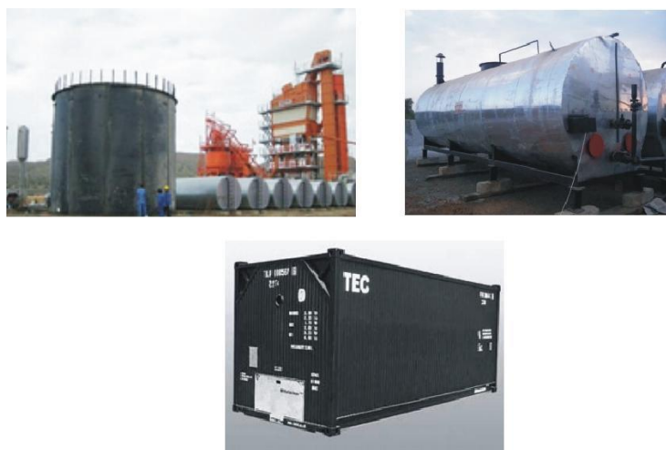
Typical bitumen storage tanks are pictured above
