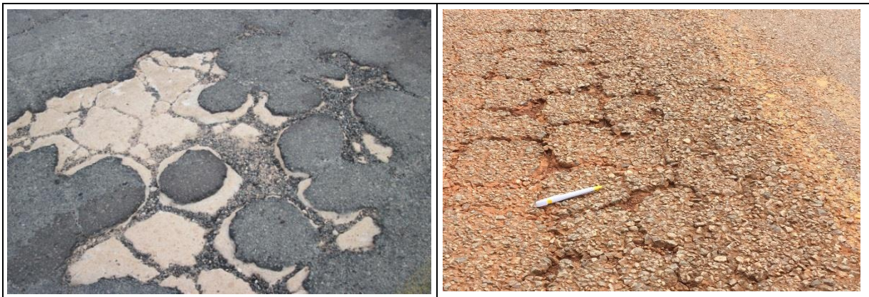
Figure A.6 Examples of Cemented Base Layers in an EG4 Stage of Deterioration
