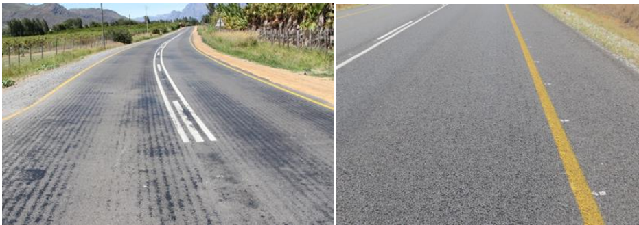
Figure F 13 Effects of Poor Transverse Distribution
