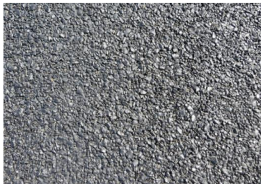
Figure H 6 Non-Stripped 14/7 Double Seal Texture
