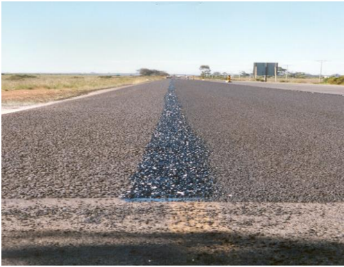
Figure F 24 Additional Joint Over Spray
