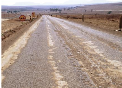
Figure D 10 Poor Performing Single Seal
