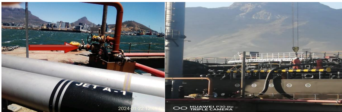
Figure 3 – Ship to shore discharge via a pipeline using a fixed quayside connection to an onshore storage facility. On the left the red arrow points to the shore pipeline connection flange and on the right the shore pipeline is connected, via a flexible discharge hose, to the vessel alongside at the Tanker Basin in the Port of Cape Town. (Images courtesy of Rubis Asphalt South Africa)
