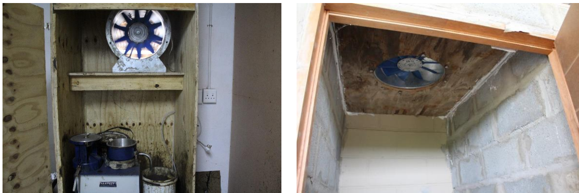
Figure 4: Even if these fans are of sufficient capacity to clear vapours from the atmosphere, a negative effect would be that the harmful vapours are actually drawn up and through the breathing zone of the operator
